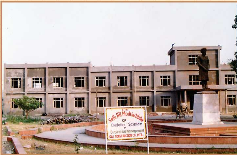
Construction of H. R. Modi Centre of Computer Science & Business Management in progress
